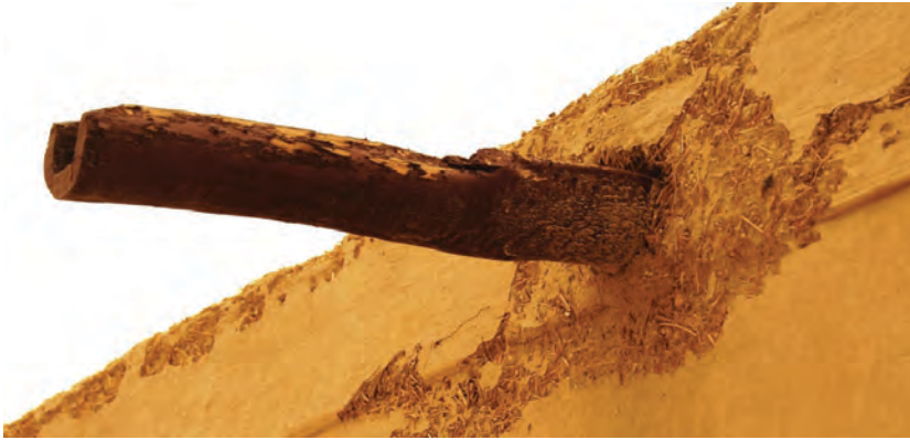
Figure 22. Gutter made out of wood in the newly renovated Jawatha Mosque. Source: Author
