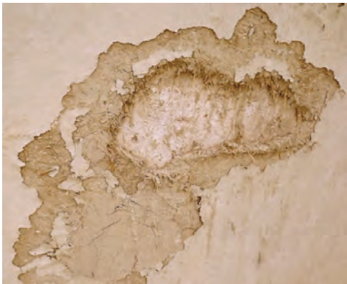
Figure 23. Earth plaster falls out. Source: Author
