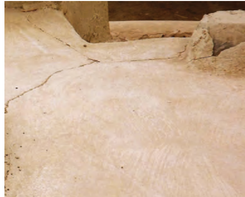
Figure 24. Cracks on the roof earth plaster. Source: Author.
