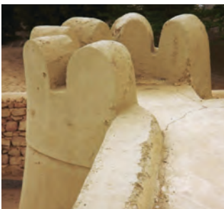
Figure 19. Parapet wall of the bastion of Jawatha Mosque. Source: Author.
